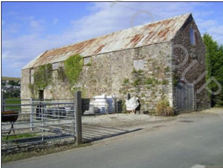
The mill from the north east showing the 19th century Extension with cart door onto the road and date stones for 1861 and 1598 in the wall above
