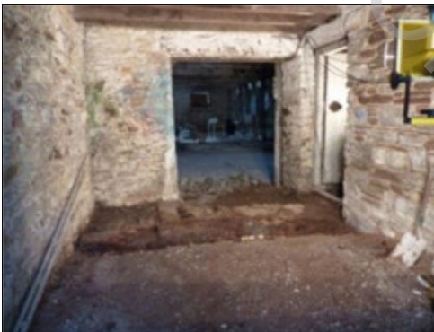
Looking south through the Extension Area A. Door D2 to the right; door D3 ahead. Excavated area on threshold of D3
