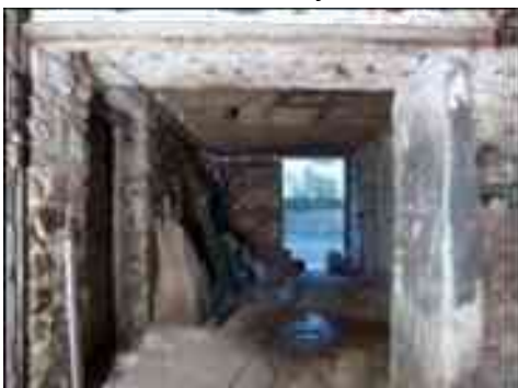
Looking north from door D3 through Area A out to the road
