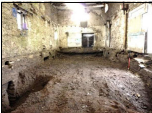
Looking north: ground floor joists removed. Showing the surface of the clinker fill in the Basement at the south end
