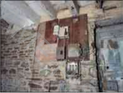
Electricity board in Area B next to the ground floor doorway D2
