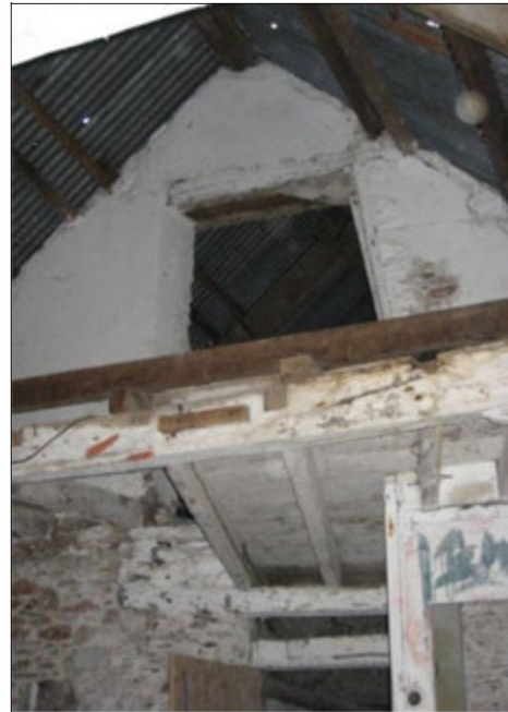
Looking north on the first floor; stairs to right, door D5 and sack ramp above
