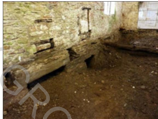
Looking northwest: S3 (left) and S4. Joists J3 and J4 removed, J5 beyond. Blocked sluice controls F2 & F3 in the wall above
