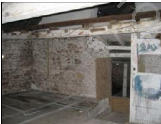
First floor looking north west. Sack ramp from door D4 to the Extension with sack ramp to door D5 above
