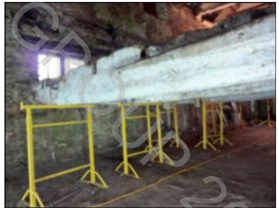
First floor beams cut down with Beam 5 in foreground. Note the iron hasps in the side and underneath which would have been used to lift the mill stones for dressing.
