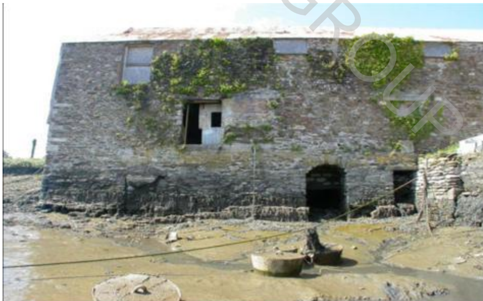
The East wall at low tide showing the sluice openings at Basement level.
