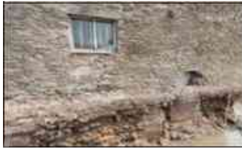
West face foundations and blocked sluices
