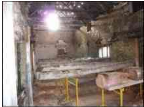
First floor beams cut down looking south with rot-ten stumps retrieved from the wall in the foreground
