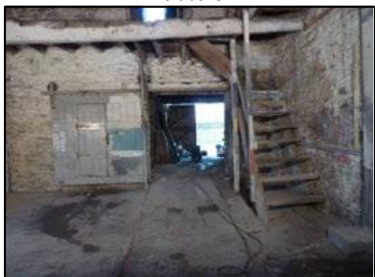
Ground floor looking north to stair. Door D3 with 20th century sliding door and D1 beyond
