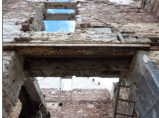
Detail of Doorways D4 above and D3 below showing steel lintel and re-used mill lintel. Looking north
