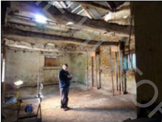
Ground Floor looking south with Beam 5 showing an iron hasp on the underside in the foreground
