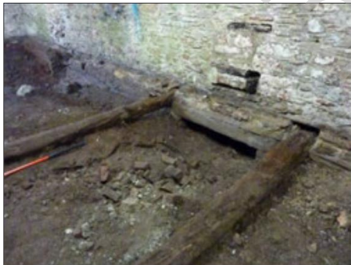
Looking south west: ground floor joists, J3 (with scale) and J4 on each side of sluice S3 lintel. Blocked sluice control F2 in the wall above
