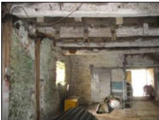
Ground floor looking north with Beam 4 in foreground. Remnants of a wooden hopper from the upper floor showing as sawn off vertical timbers
